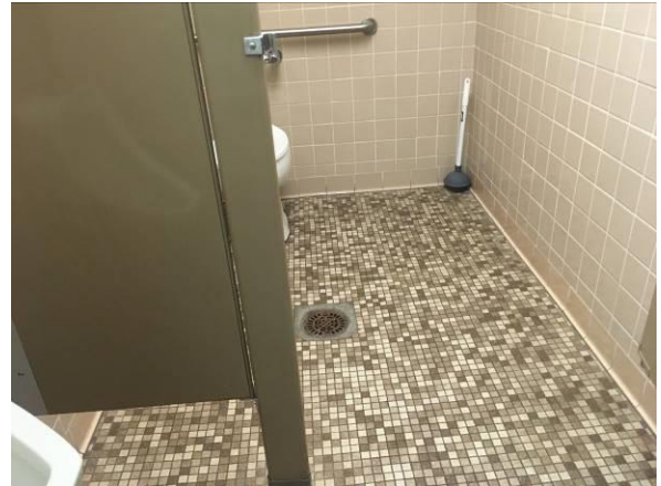
Photo #14 View of one of multiple floor drains located throughout the on-site buildings.
