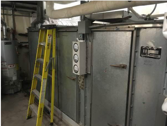
Photo #13 View of boiler located in the sub-grade boiler room of the Bergere House.
