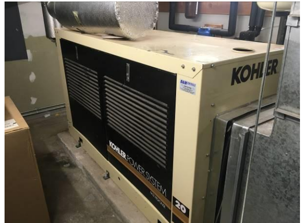
Photo #10 View of natural gas-fired generator located in the sub-grade boiler room of the Bergere House.
