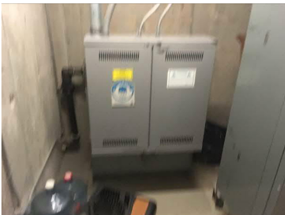
Photo #11 View of elevator mechanical room located in the basement area of the Bergere House.
