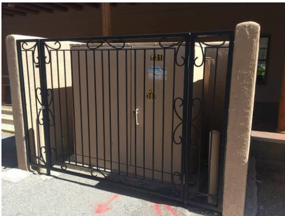
Photo #15 View of one of three pad-mounted transformers located in the southern and northern portions of the site.
